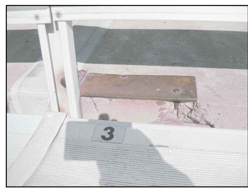
18b TYPICAL STEEL PLATE CONDITION (SOME VARY)
