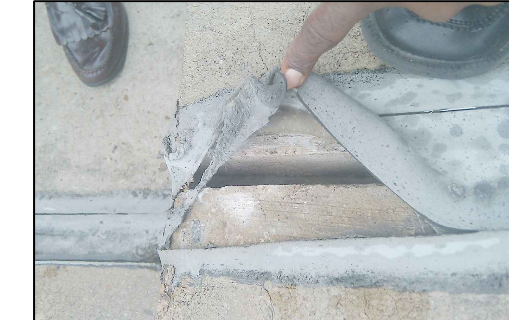
9 EXIST. EX. OF EJ @ TREAD/RISER CONDITION REQUIRING MINOR CONC. REPAIR EFFORTS, TYP.
