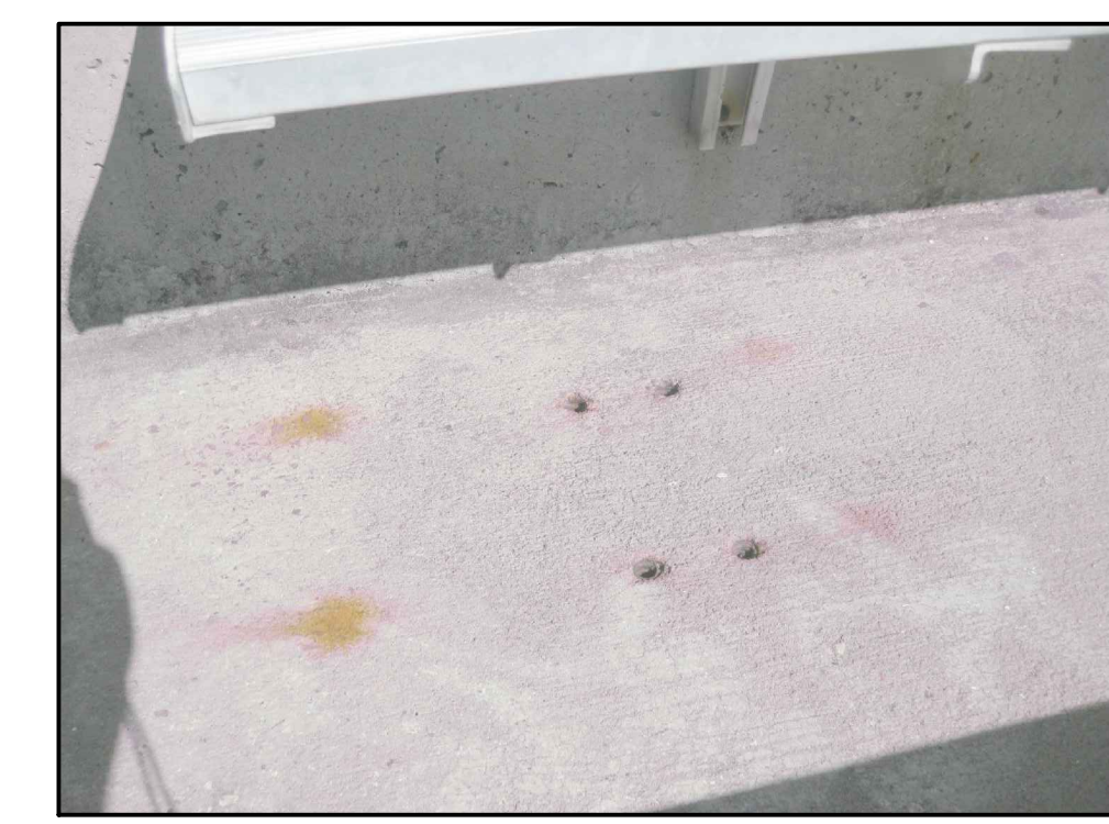
23 EXPOSED ABANDONED METAL CONDITION
